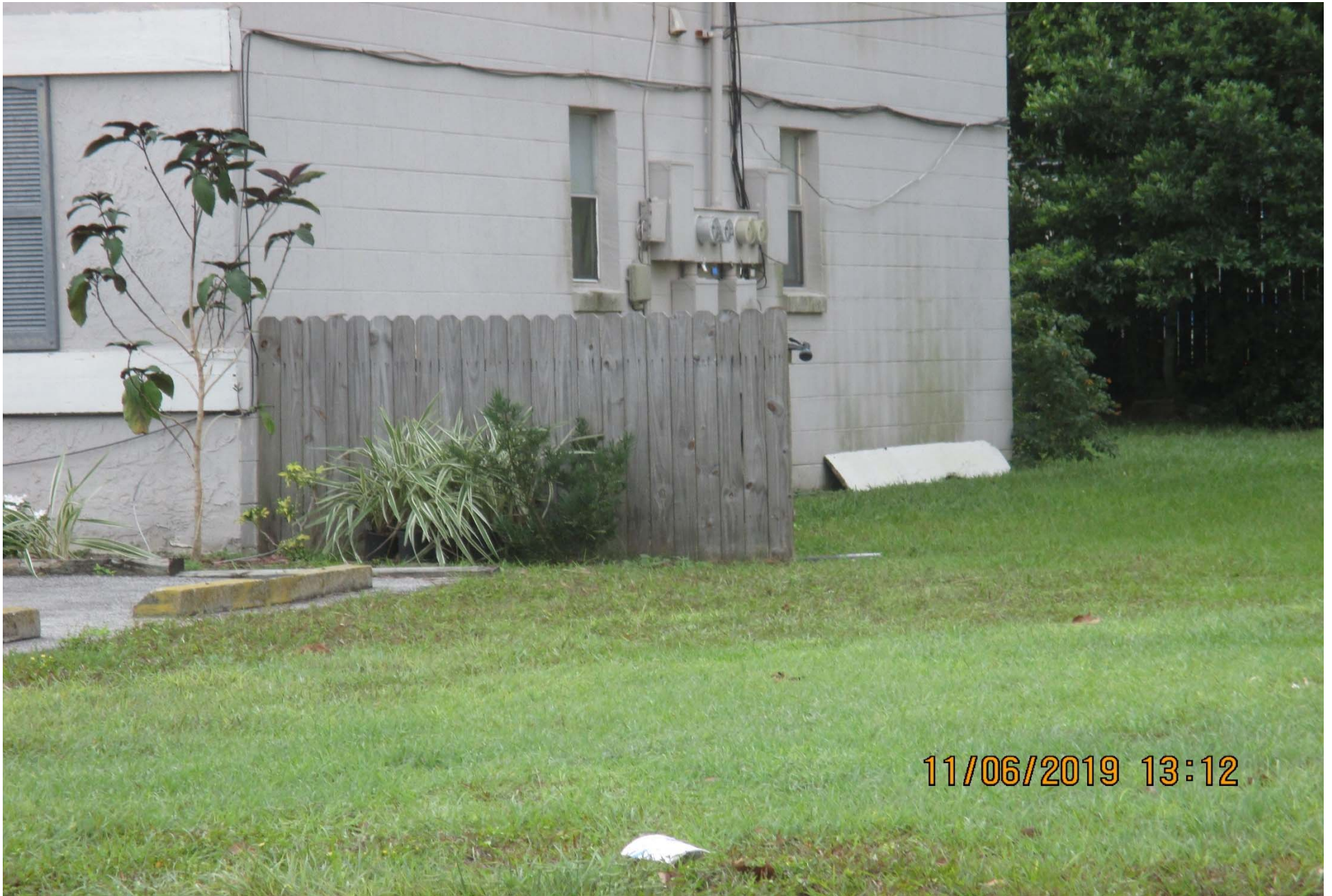
Black growth on side of the building 11/06/19
