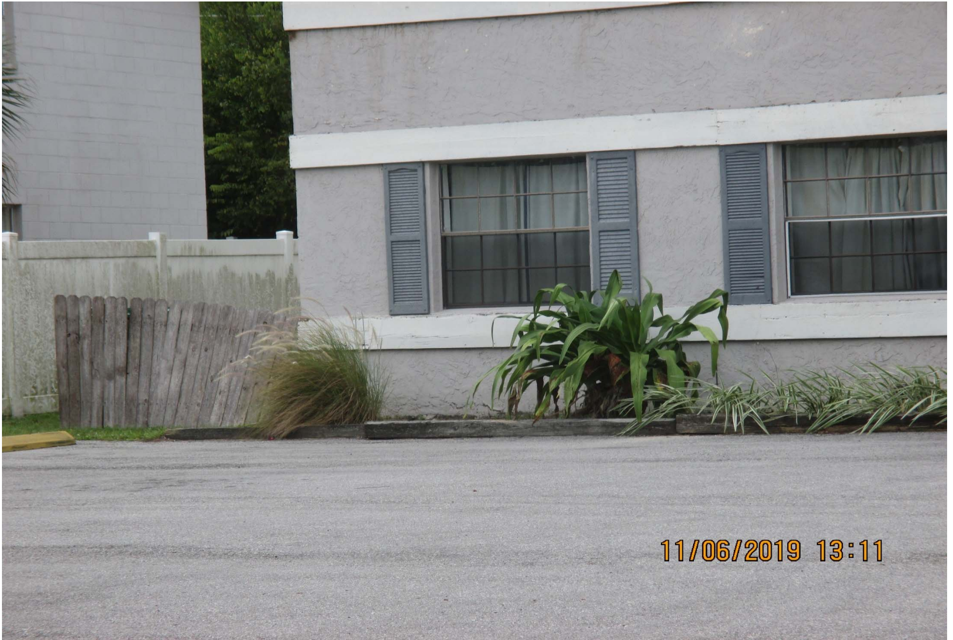
Fence falling paint chipping off of the building 11/06/19
