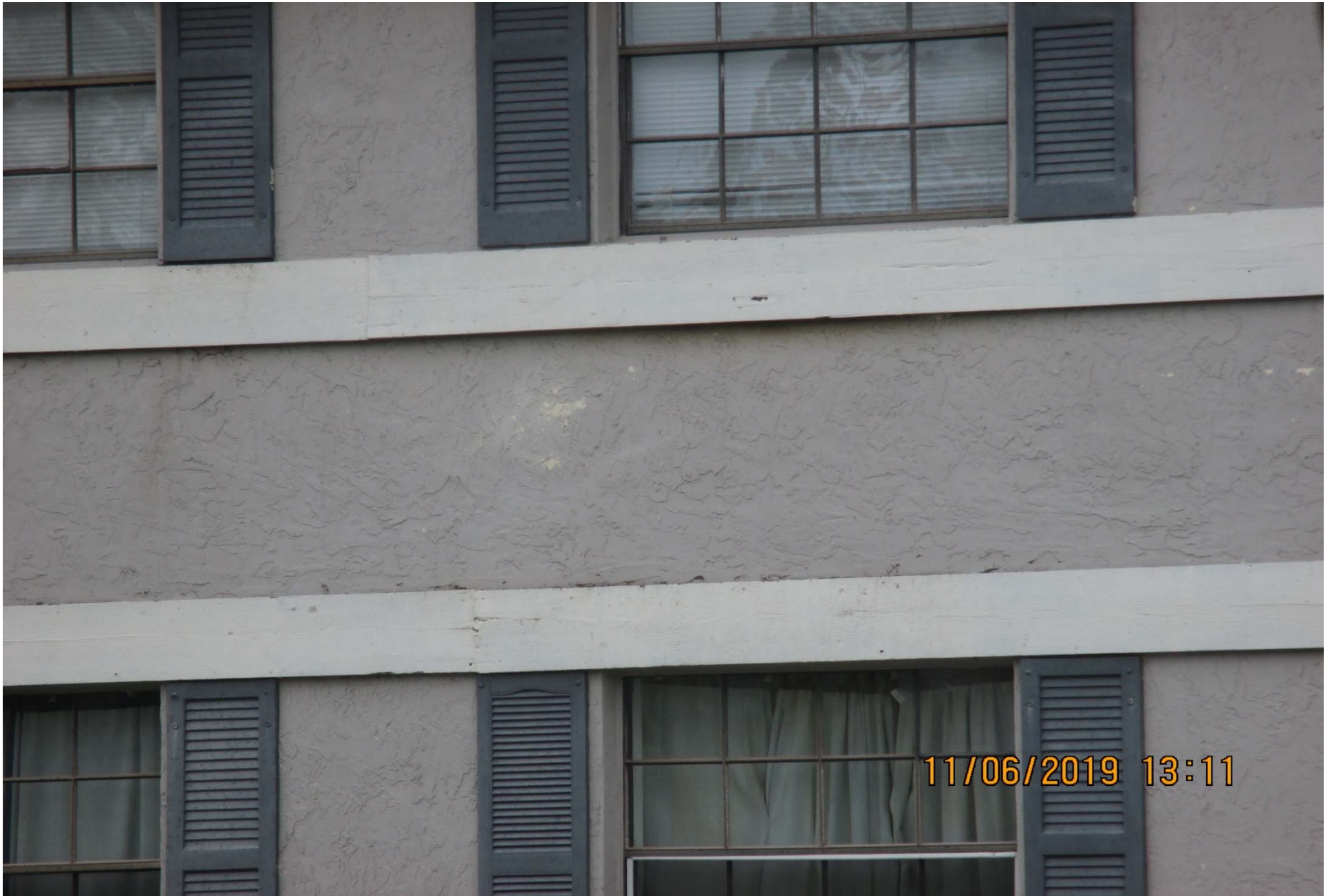
Paint chipping off of the building 11/06/19
