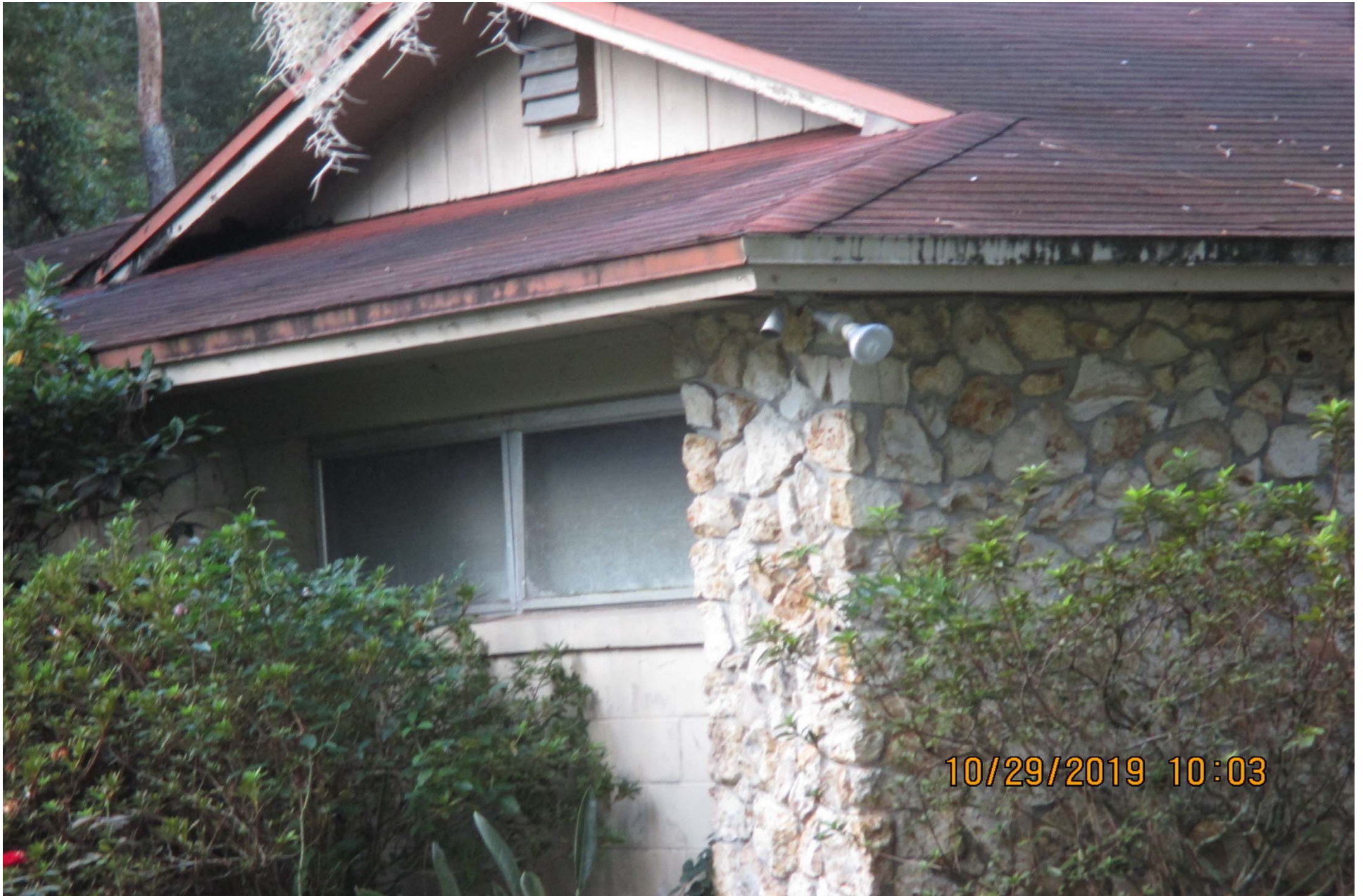
Black growth on soffit area and paint chipping 10/29/19
