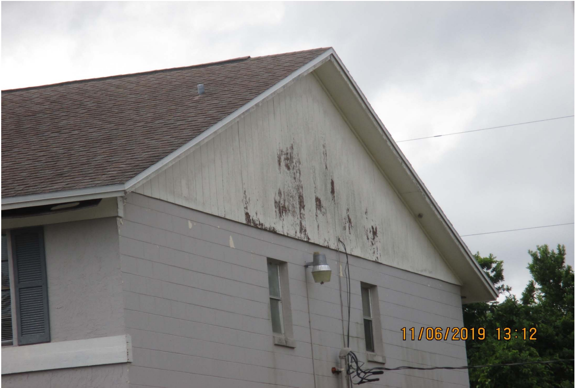
Paint chipping off of the building and soffit falling 11/06/19
