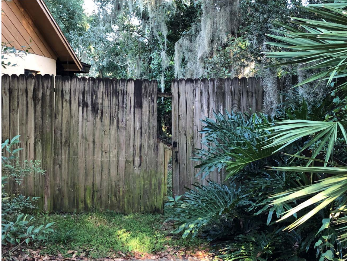
Fence in disrepair
