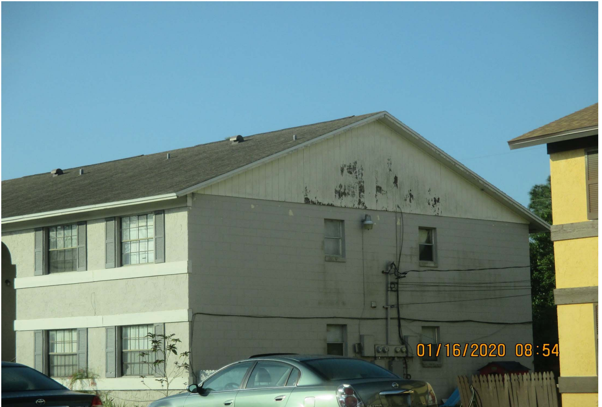
Violations not corrected as of 1/16/20
