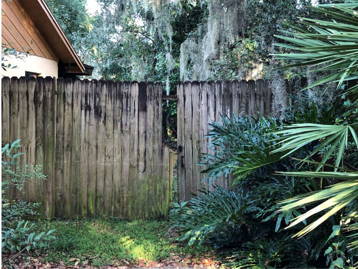
Fence in disrepair
