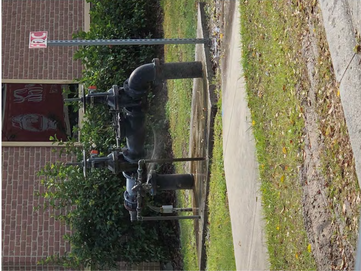
Backflow Prevention Leaking
