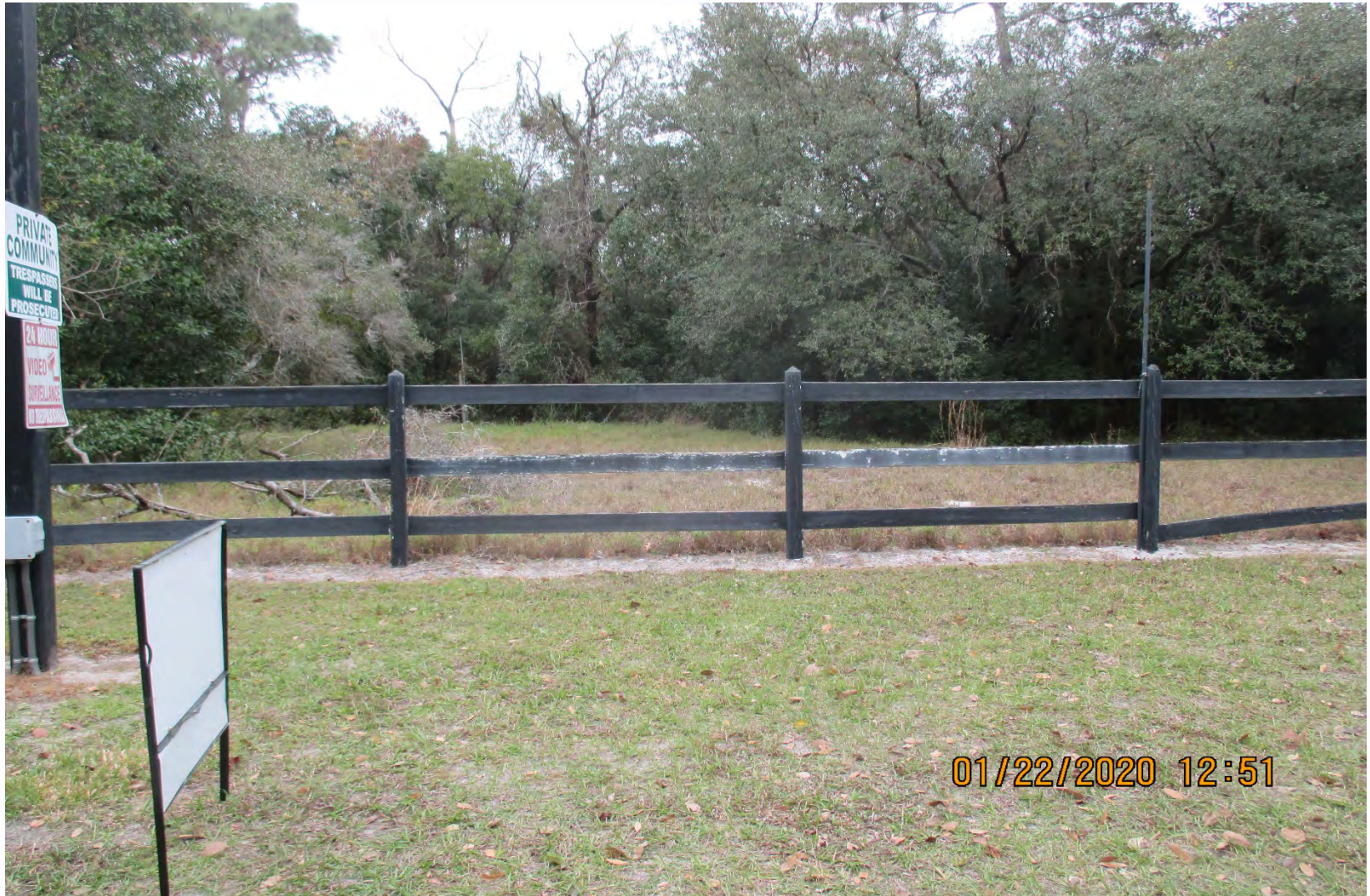
Paint Chipping Off Fence/Slats Broken 01/22/2020
