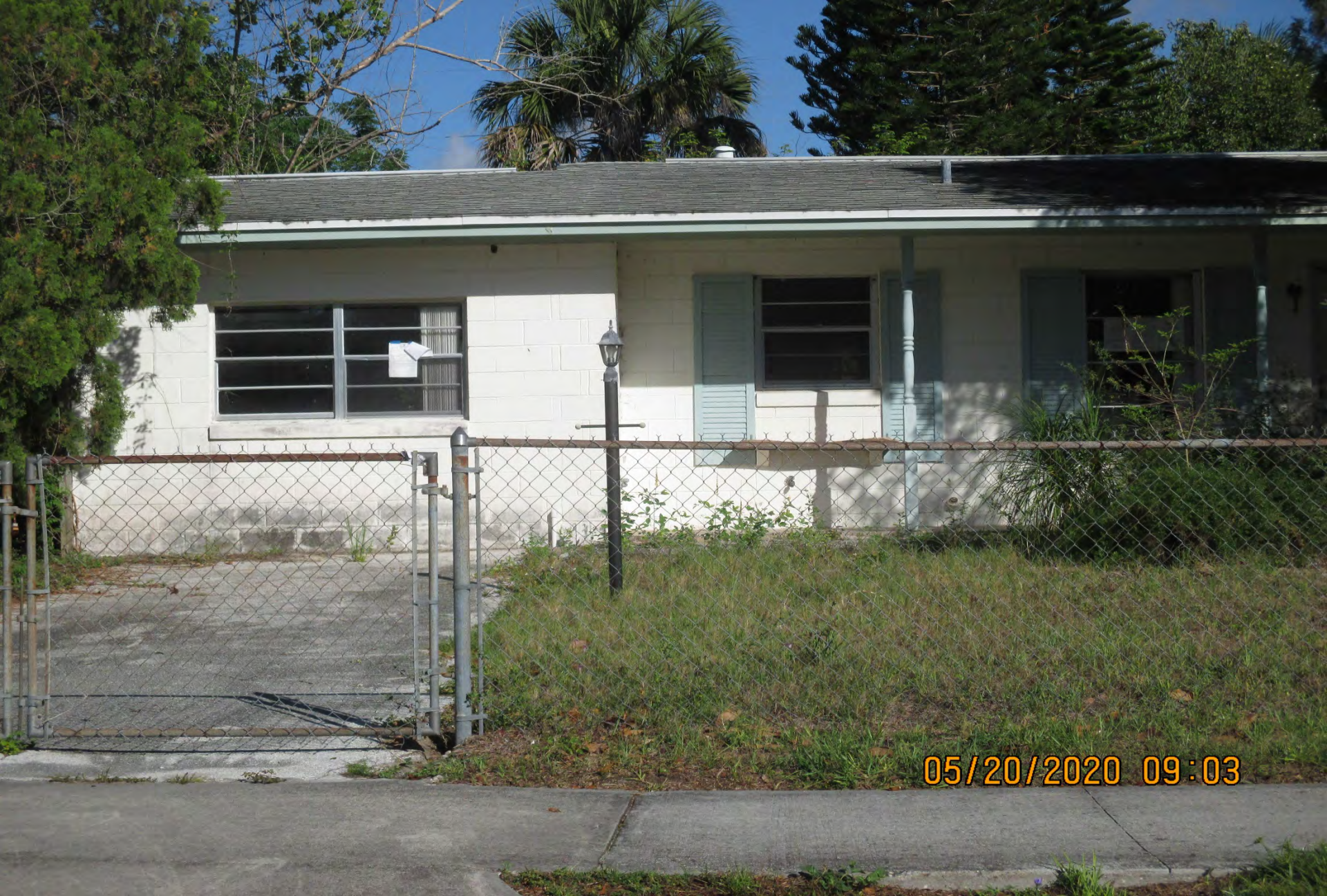
Sanitation and grass overgrown
