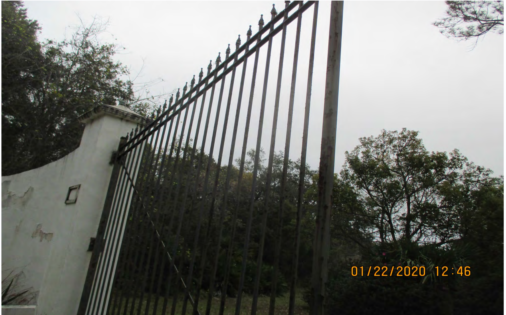
Paint Chipping Off Gate 01/22/2020
