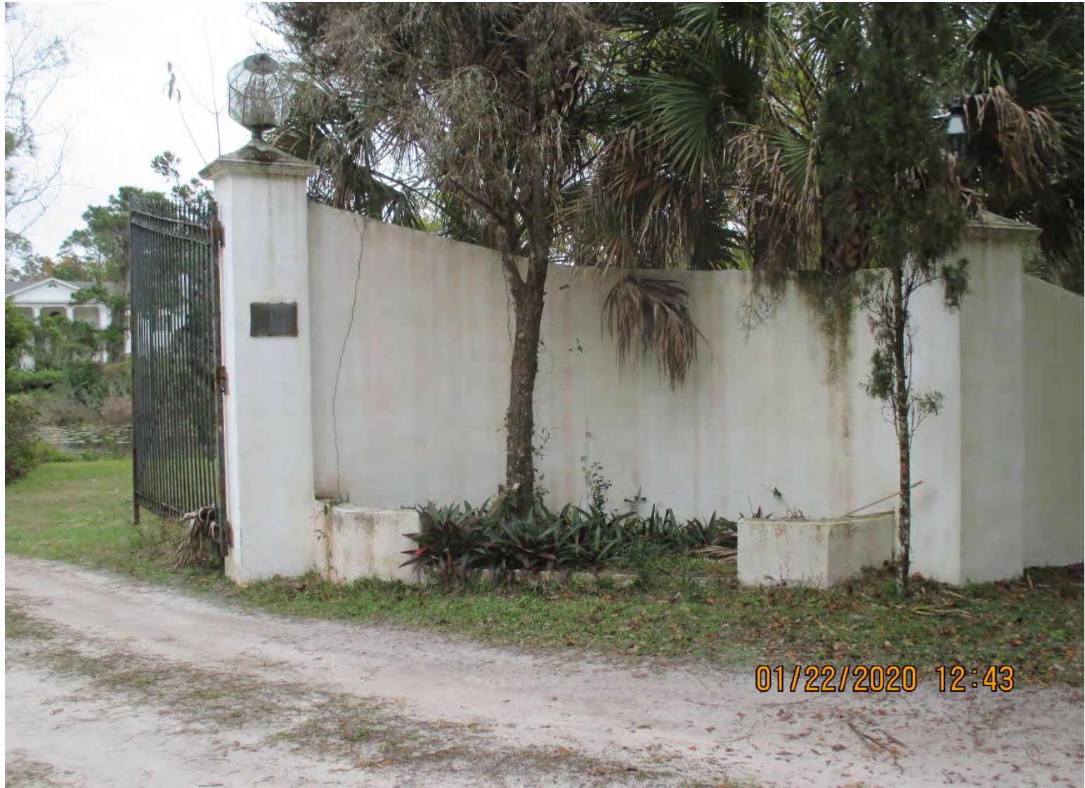
Light fixture broken/ Yard debris 01/22/2020
