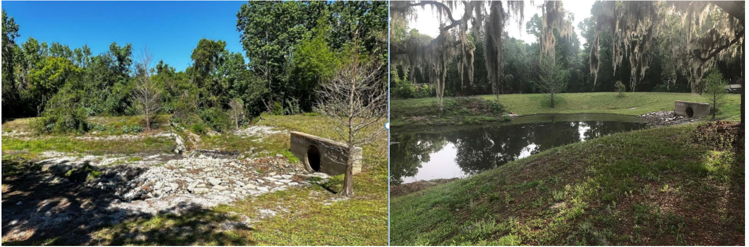
The photo on the left shows the damaged stormwater pond after hurricane Ian, the right is the pond after repairs.
