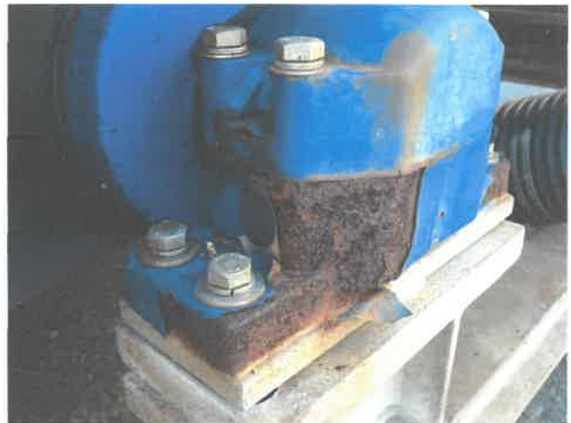
Competition, two piece split housing. Notice where the rust started..
