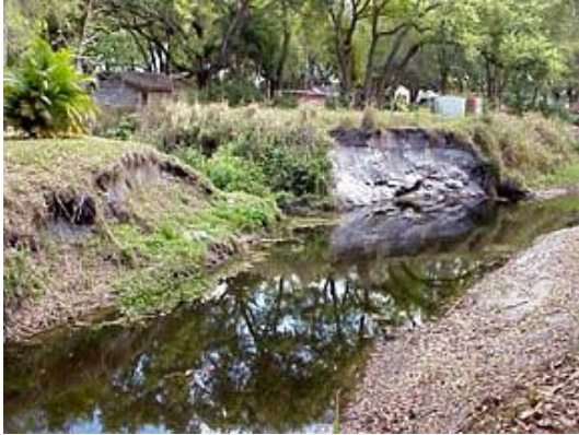
Area along the Little Wekiva River Basin where soil erosion is visible.
