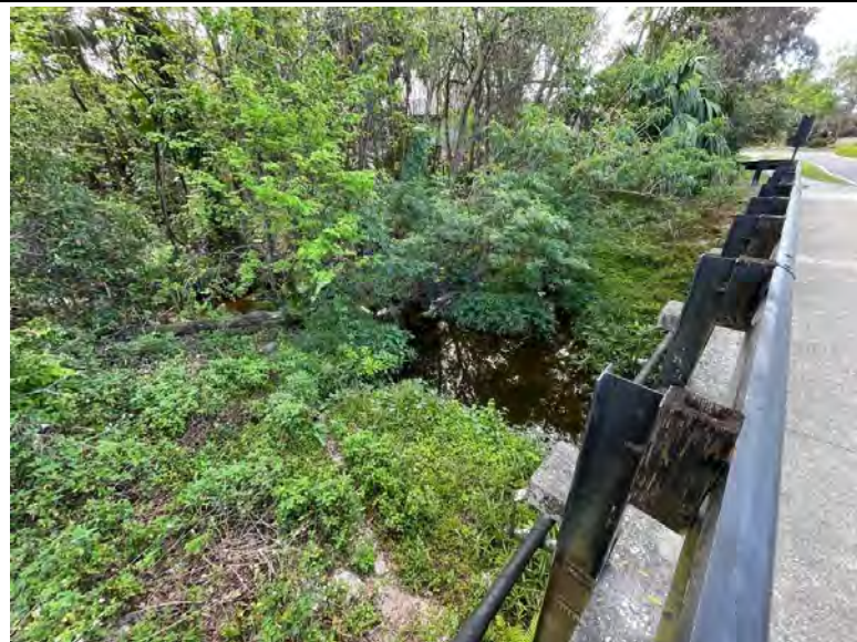
East of the Sheoah Boulevard roadway crossing (facing southeast), clear from debris
