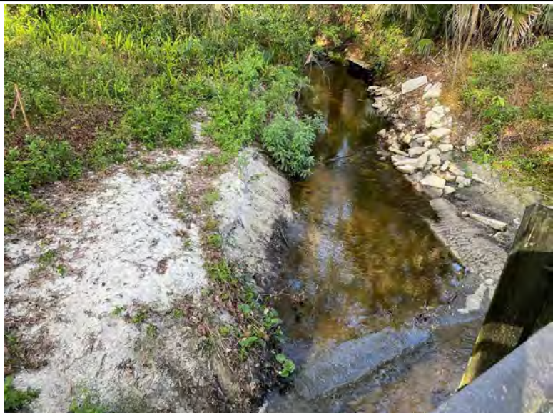
2 West of the Shepard Road Bridge (facing west), clear from debris and sediment
